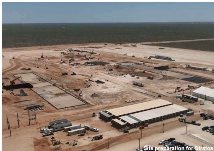
Figure 7: Stratos Direct Air Capture plant
